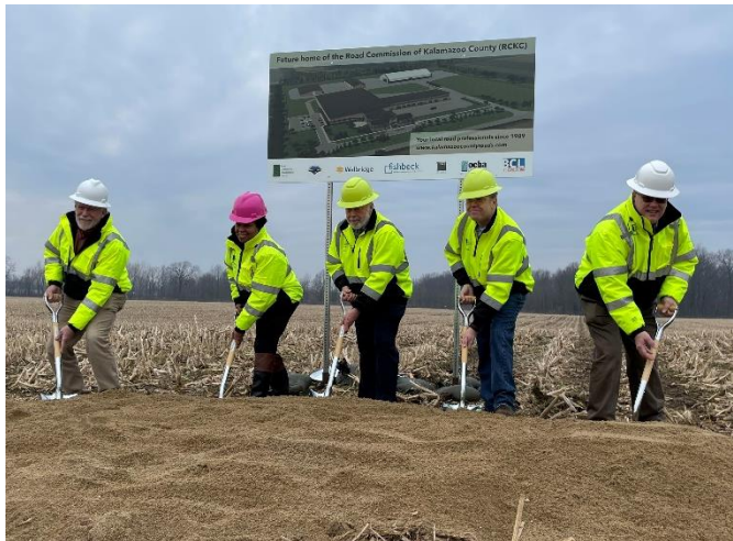
RCKC Board of County Road Commissioners break ground at the site of the new complex
